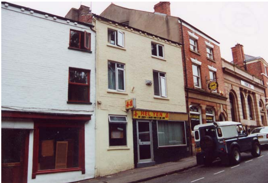
Plate 53 No. 7 Market Street : Modern Shop Front of Poor Visual Quality with pvcU Window Units at First/Second Floor Level
