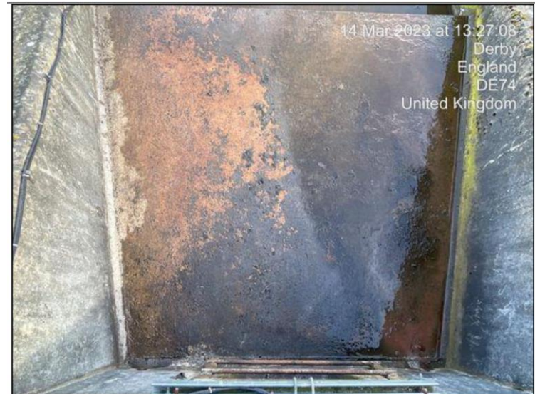
Photograph 11: Site C Gimbro Outlet.
